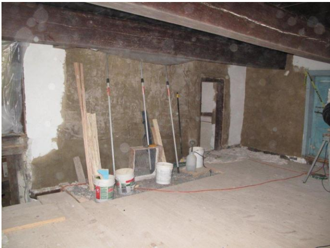
Center room with new hemlock floor, cutout for jambless fireplace hearth and partial plastering on wall
