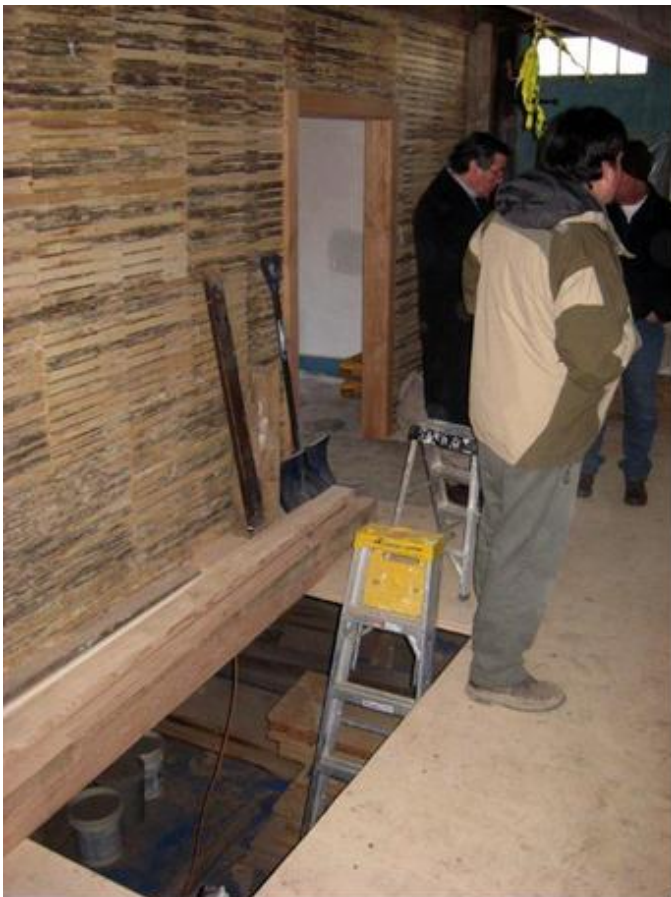
Center room showing lathed wall and door frame to south room and temporary opening to cellar
