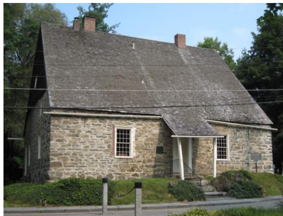
The Jean Hasbrouck House needs a new roof
